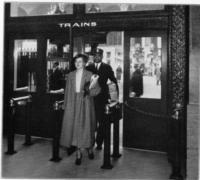
Fig. 22. Door Controlled by a PHOTRONIC Relay
